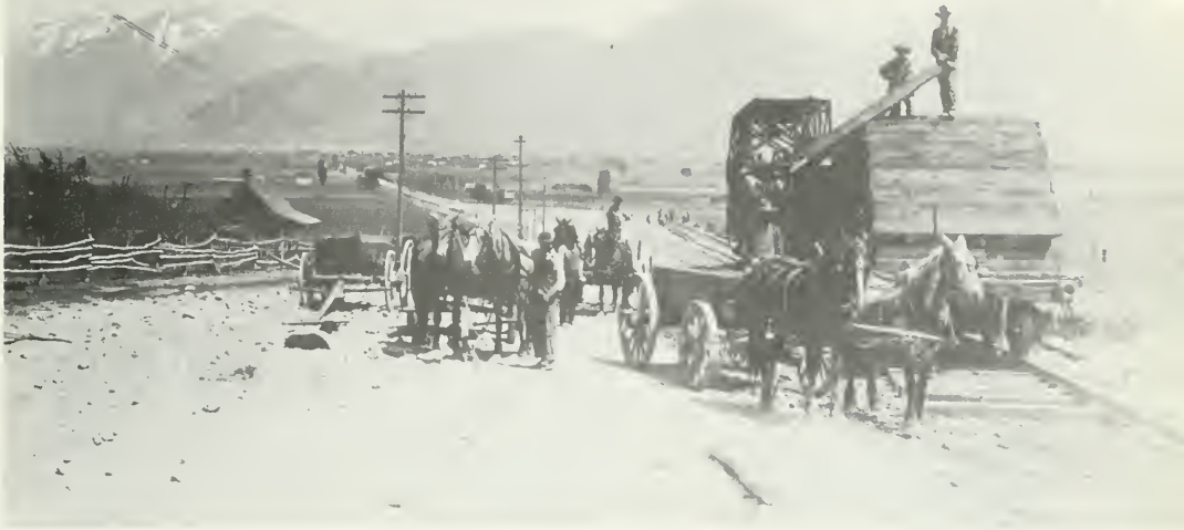
Motorized construction equipment was still in the future even during the last years of interurban development, when the Salt Lake & Utah constructed its line into Payson, Utah, on the eve of World War I. FRED FELLOW COLLECTION.
